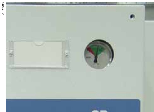
Pressure gauge indicating the pressure of the gas SF 6
