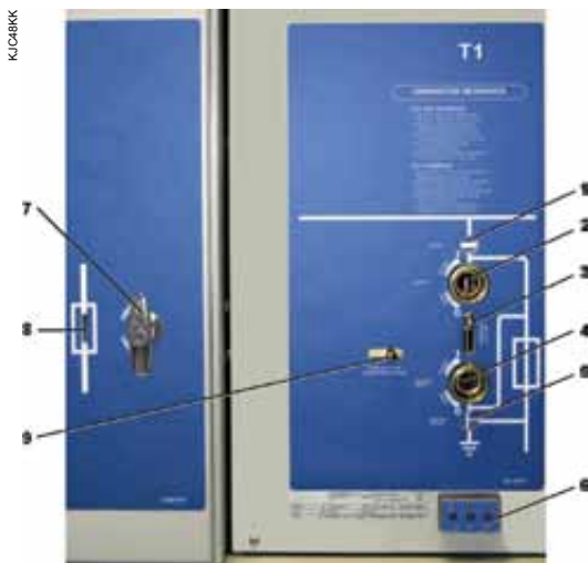
Transformer protection unit (T1) commands and controls
