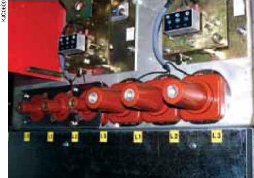
Bushing for cables connection
