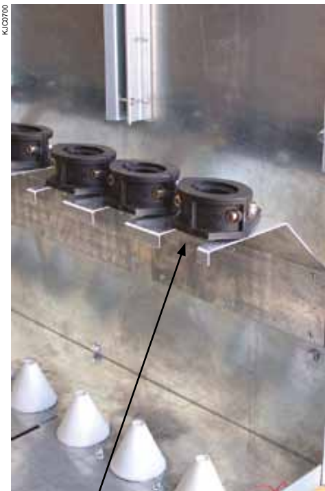
Cables clamp mounting
