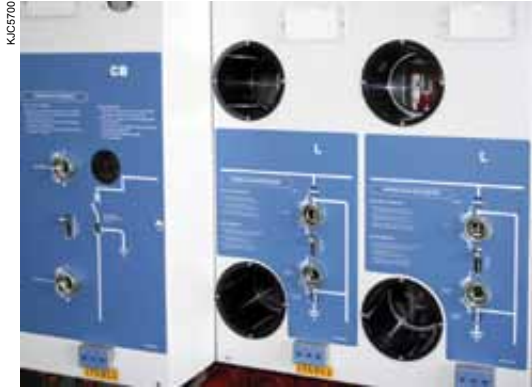
Switchgear equipped with inspection windows
